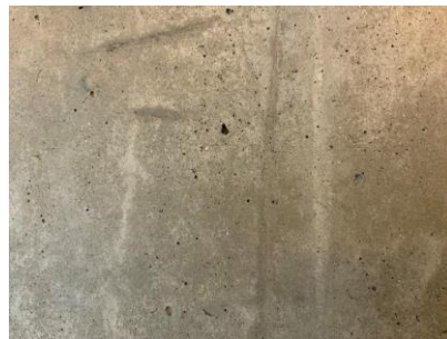
Figure 1. Surface voids on the surface of the wall
